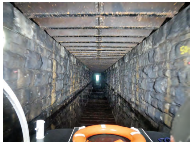
Iron revetments in the roof of the canal tunnel.
